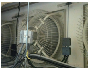
Exhaust fans for expelling heat generated by ICT equipment
